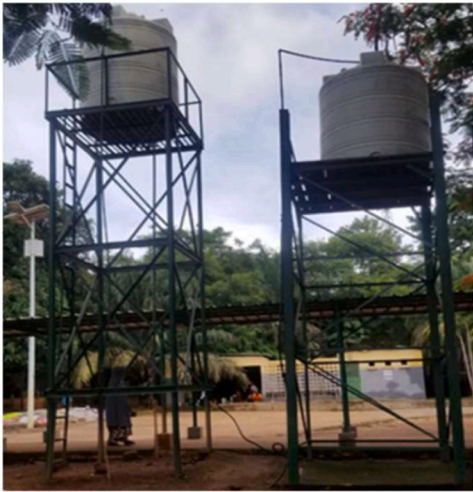
Fig. 6. Boreholes and elevated water tanks at the Faranah Region Hospital.
